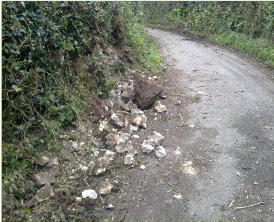
A distressing picture , sent in by Keith Legg. It shows damage caused by a large lorry from Ireland, to the banking in Colham Lane. no doubt caused by a leprechaun messing with its sat-nav. Will reparations for this damage feature in the Brexit negotiations, I wonder?
